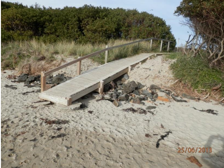
Rock revetment and walkway onto beach within 200 m west of the SLSC
