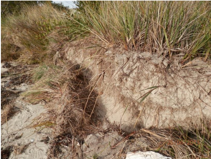
Erosion of foreshore vegetation Somerset Beach
